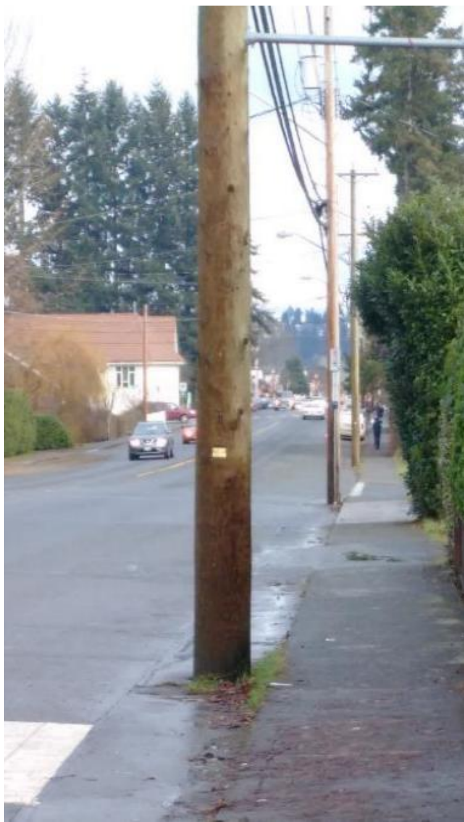
EXISTING HYDRO POLE
