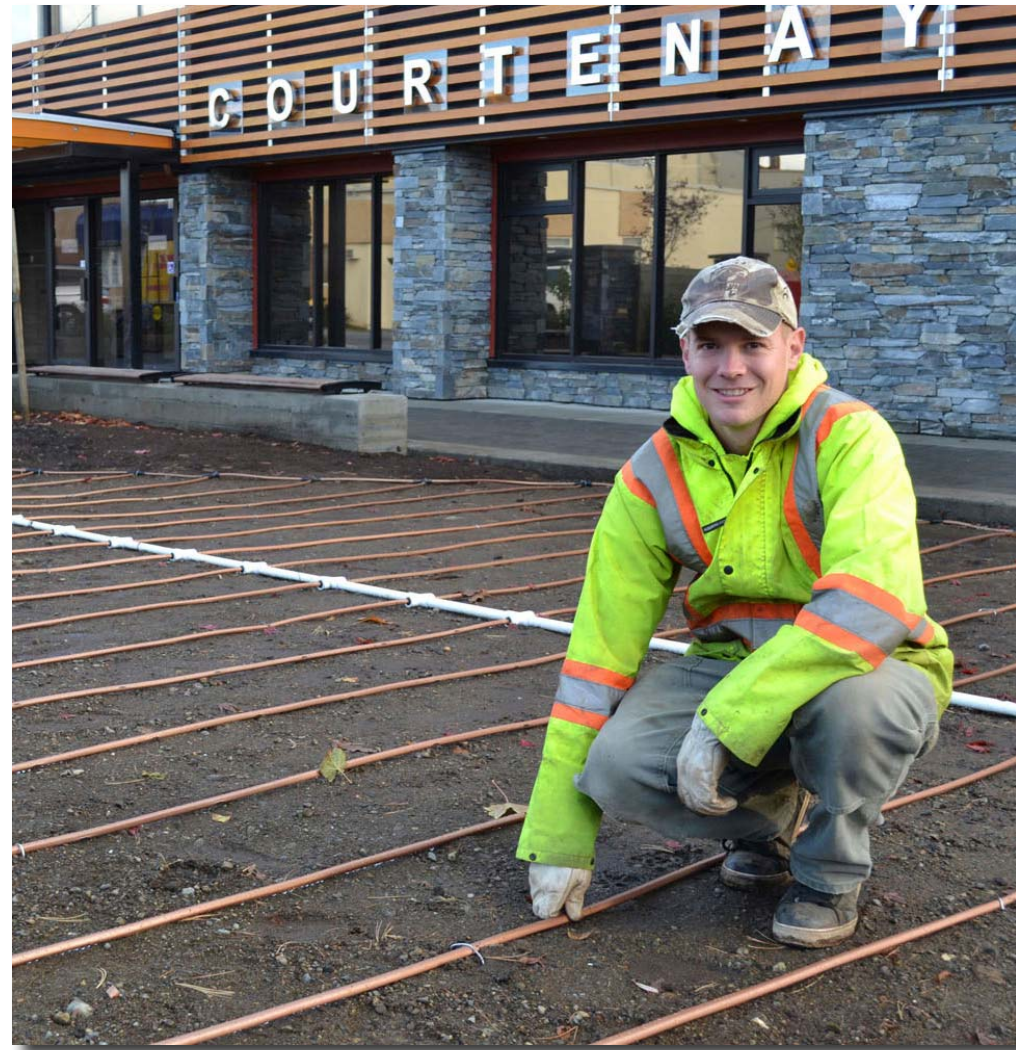
Mike Bell - City Hall irrigation
