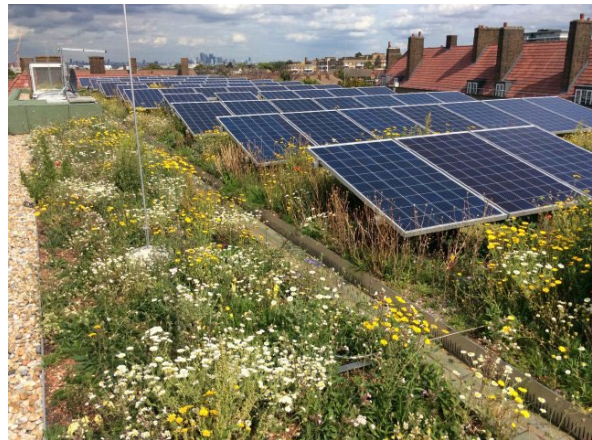
Example of solar photovoltaic panels being incorporated with greenroof elements (guideline 88 and 89).
